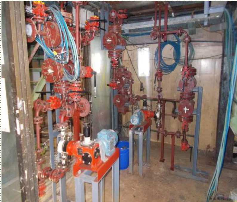
HSEF: tanks and piping
