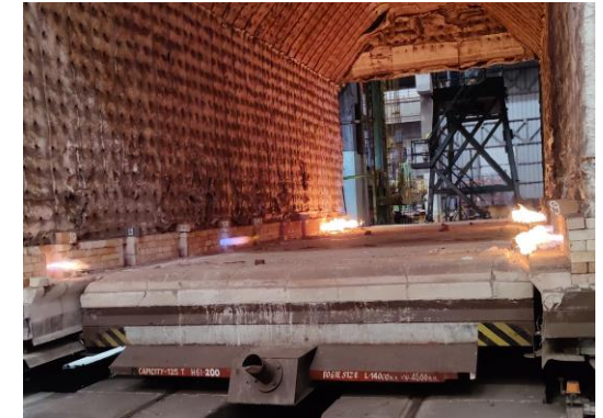
15% H 2 blended with NG used in Furnaces in manufacturing shop
