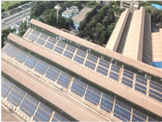
Powered by Rooftop Solar Plant
